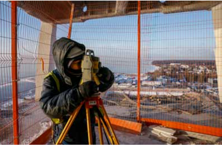
In winter the metalworkers were in the freezing cold at the construction site, nevertheless while taking measurement they had a gigantic vista.
