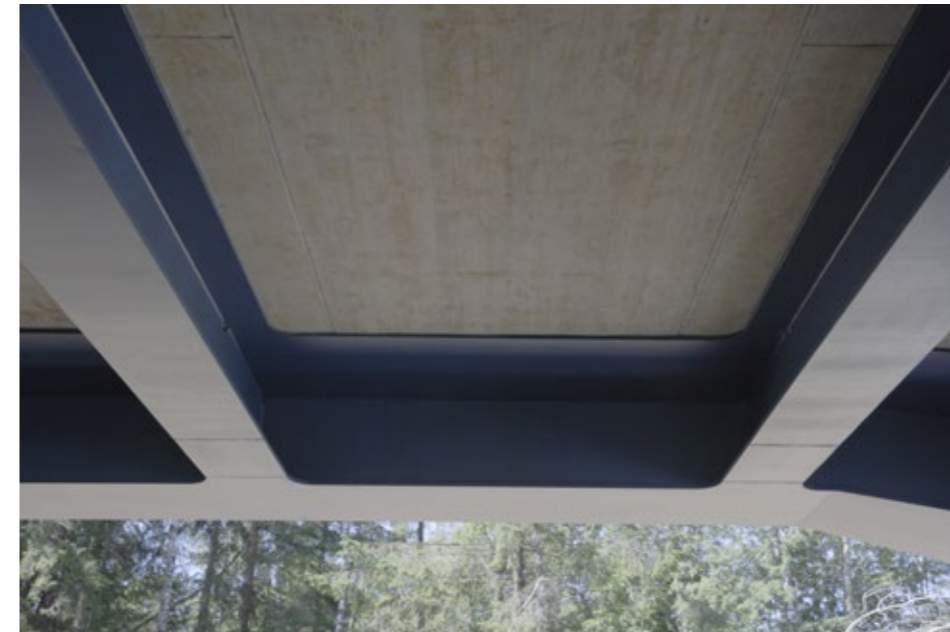
Immediately on the steel structure, the carriageway slab was concreted as in-situ concrete construction. For this purpose, a rough sawn formwork was contracted in between the steel beams.
