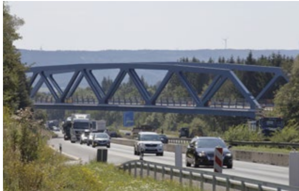
Over a weekend in August, the bridges were installed and on Monday the traffic rolled over the A45 again.
