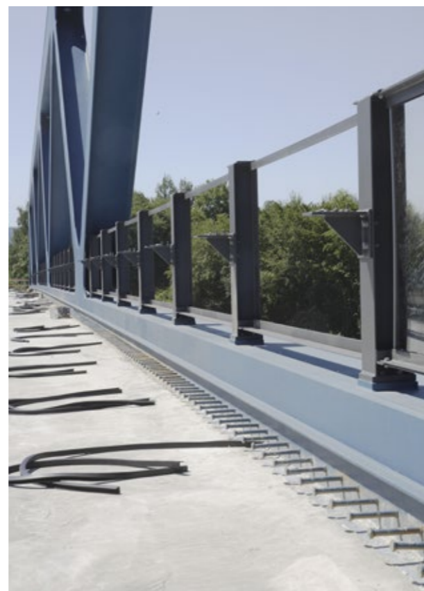
The concreted side roadway banquettes are connected to the bridge body by the outstanding reinforcing steel.
