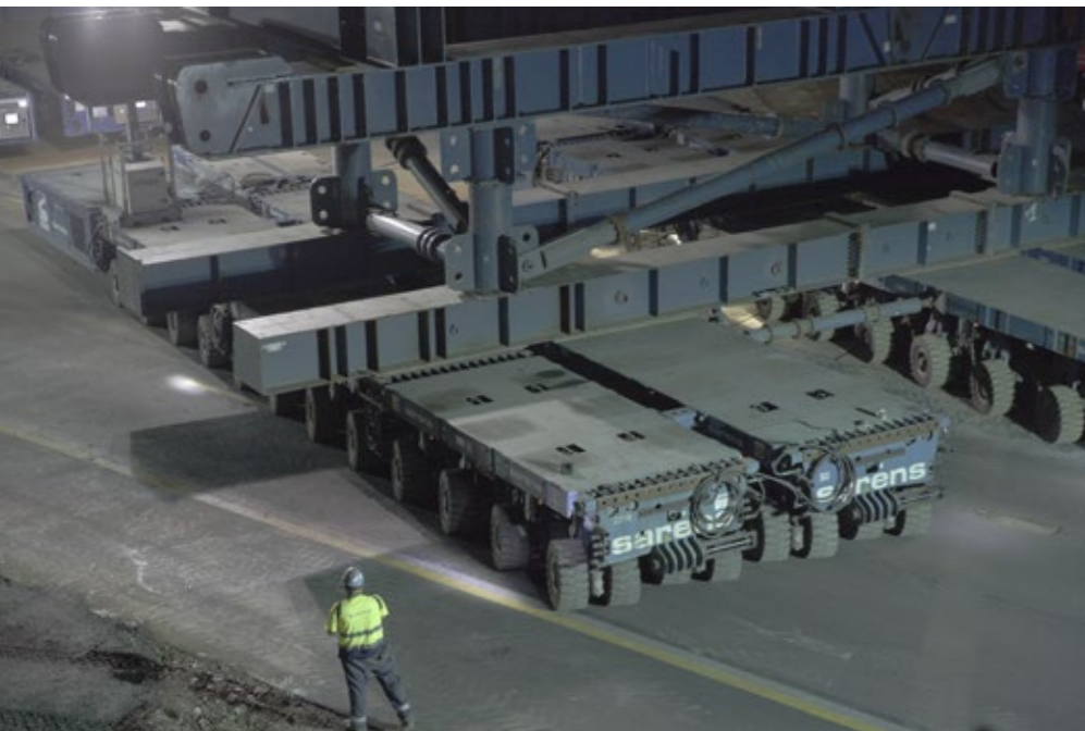
Positioning of a bridge with SPMTs. The workers with the safety vests control with radio remote controls once the front and once the rear unit of 8 vehicles connected together.
